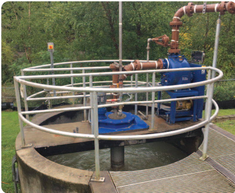
Piney Creek DSP10 – 7 MGD
