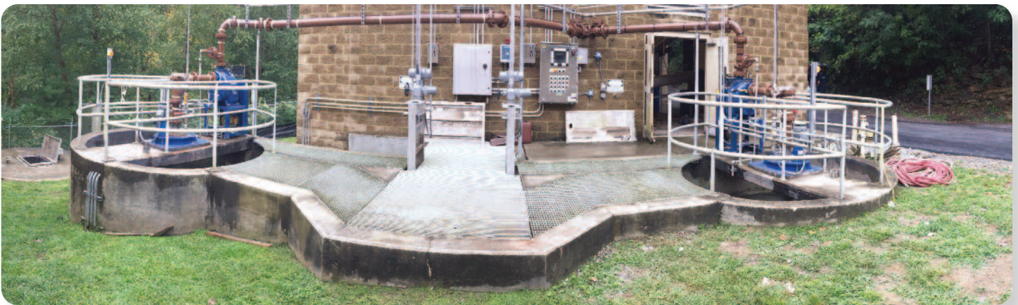
Piney Creek WWTP – Beckley WV
