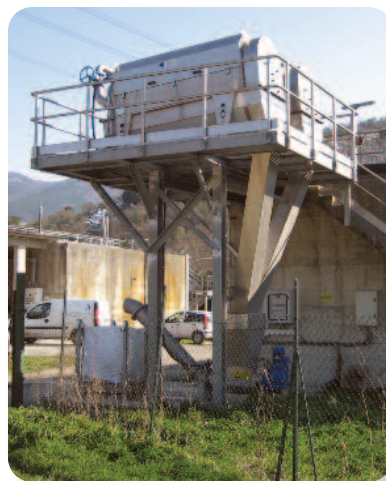
Two Flo-RotoDrum screens discharging to a Flo-WashPress.
