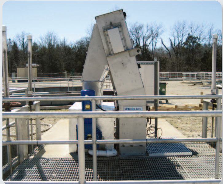
Flo-MultiRake Fine Bar Screen with 6 mm bar spacing installed at a 90° angle.
