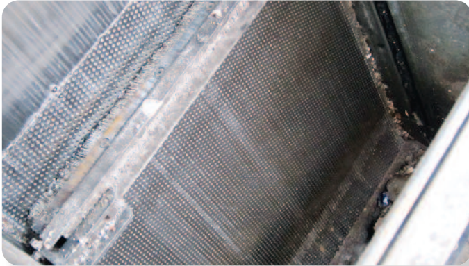
Perforated media attached to dead plate.
