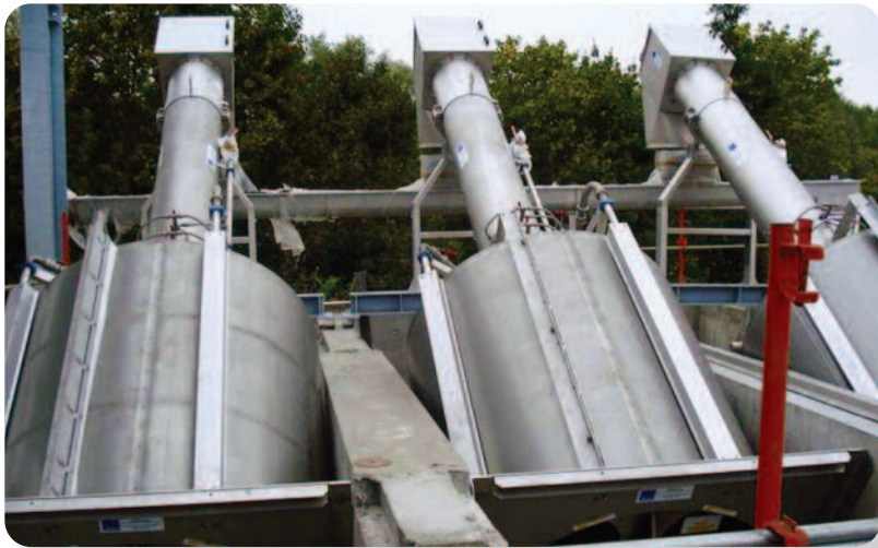
Three - FD-MBR2000 5 MGD Per Screen - Orleans, France
