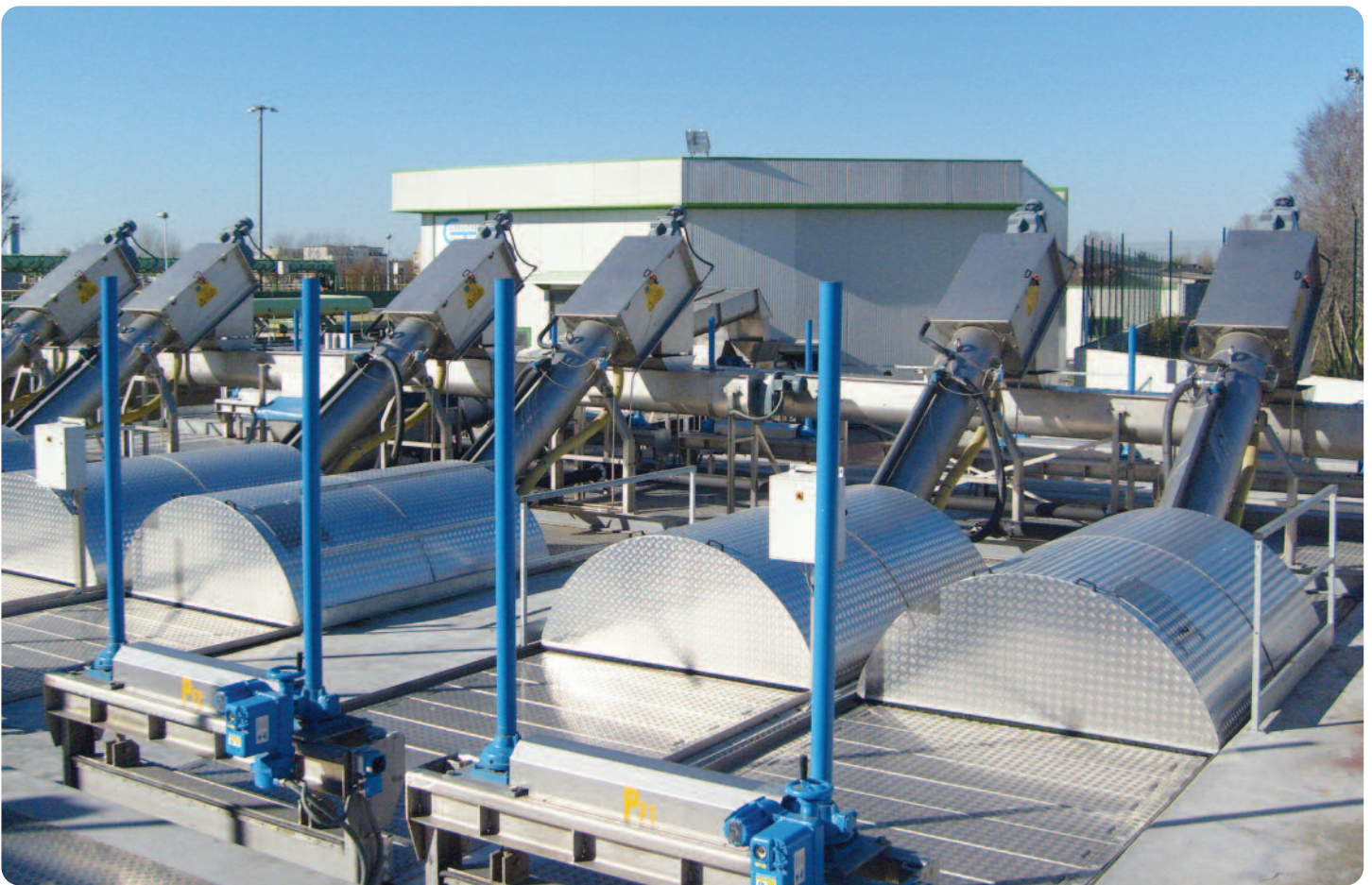
Six FD-MBR2000 10 MGD Per Screen - Brescia Italy
