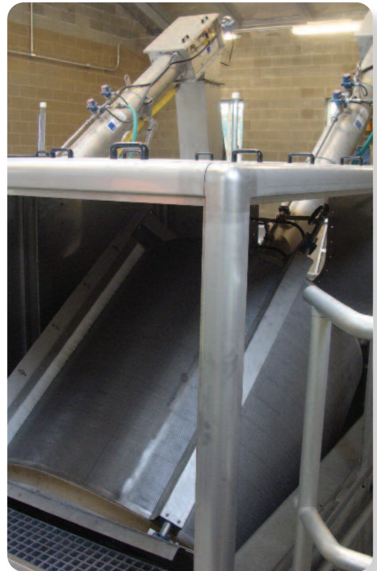
Two FD-MBR1600 6 MGD Per Screen - La Center WA U.S.A.
