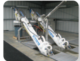
12 - Flo-Drum Units with freeze protection in Washington State
